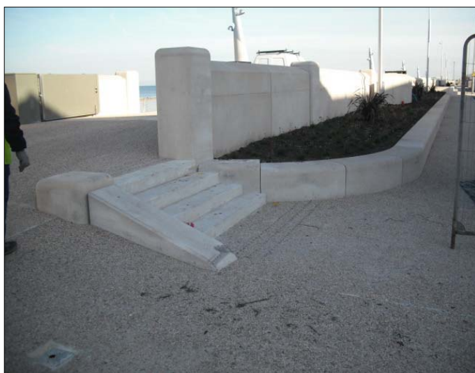
View looking up the vehicular access ramp and pedestrian access steps at the southern end of the works.
