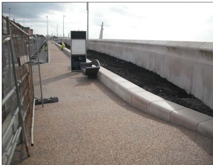
View looking south of the works from Victoria Road on the highway side of the sea wall.
