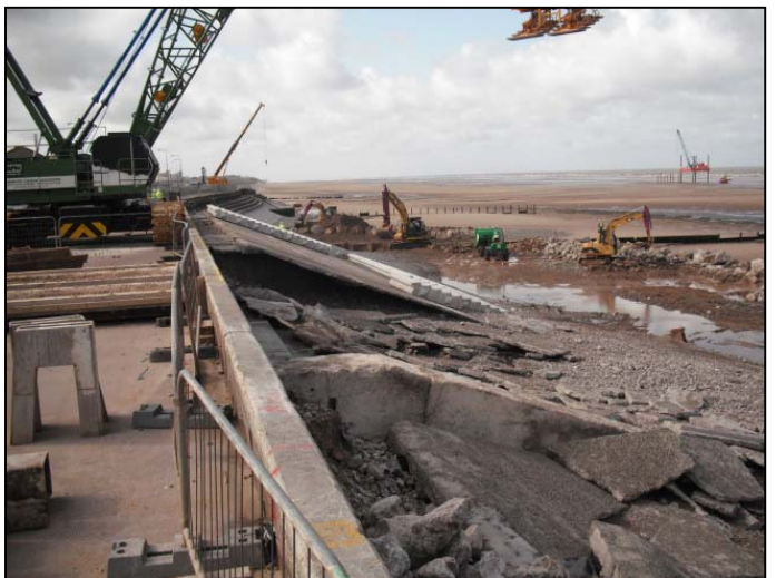
Panels 7 and 8 completely demolished and washed out.
