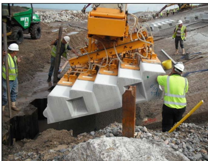
First unit being lifted into position using the vacuum lifter. Female 'joggle' can be seen on the face of the unit.
