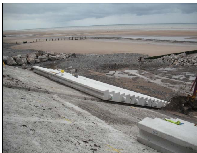
Four rows of panel 10 units complete. Male 'joggle' can be seen on the face of the units.
