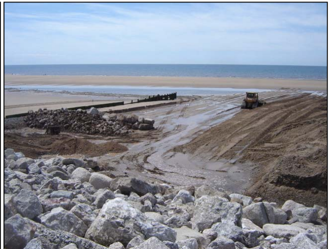
Beach level reduction continuing with rip rap being placed just west of the toe line to protect the works.
