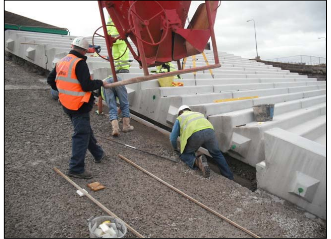
One of the central spine beam concrete base being prepared between panels 9 and 10.
