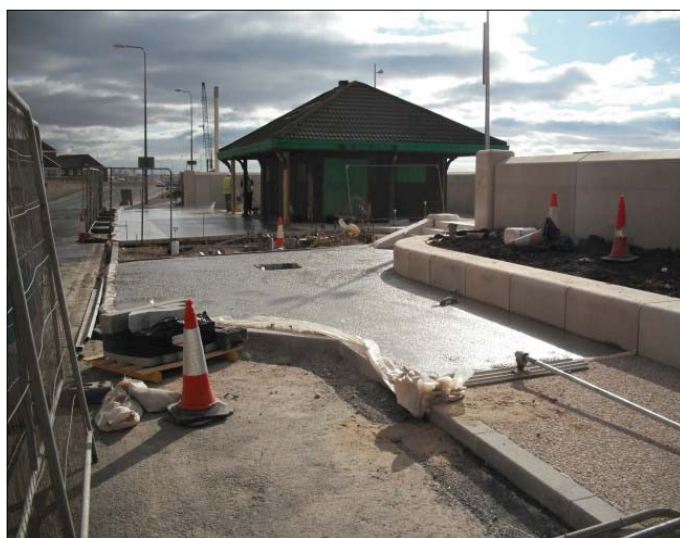
Footpath in situ pavement slab being poured around pumping station at southern end of works.
