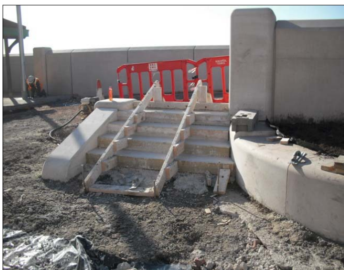
In situ concrete pour to pedestrian access steps adjacent to vehicular access ramp at southern storm gate.
