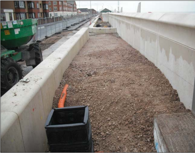
Pedestrian access ramp being filled and compacted to level ready for pavement slab.
