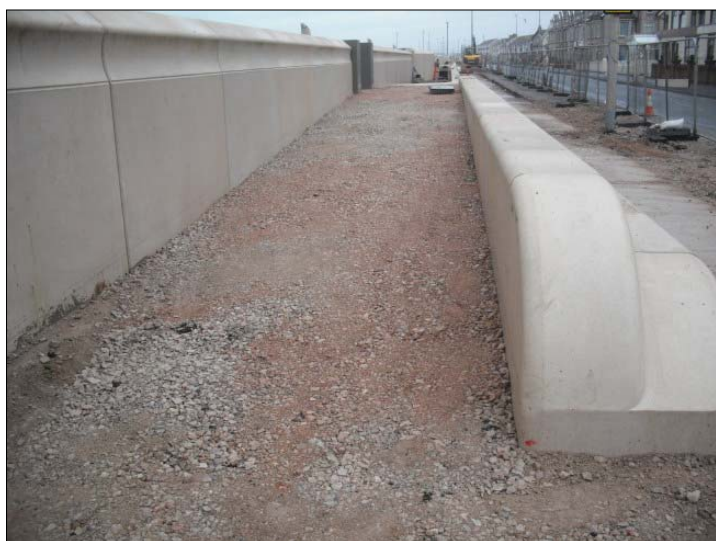
Combined pedestrian access ramp and steps on the highway side of the sea wall filled with stone and compacted to level ready for pavement slab.
