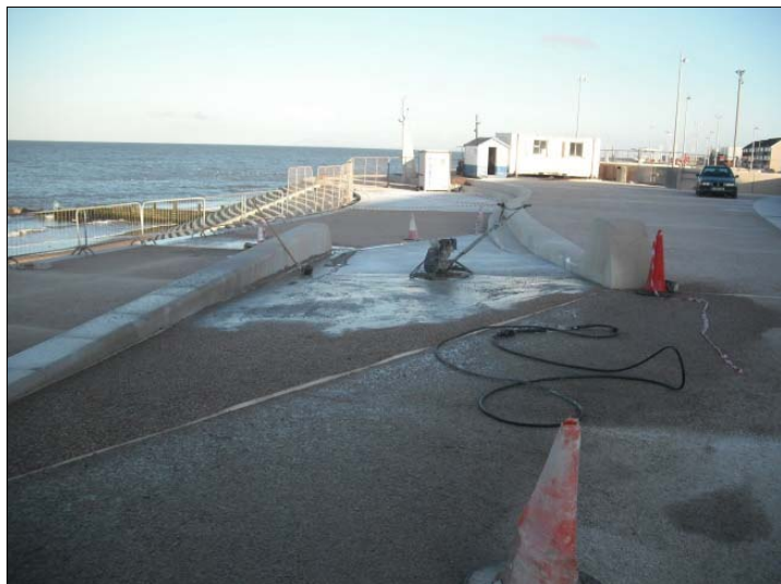
Retarder on last two pours of pavement slab being washed off leaving an exposed aggregate finish.
