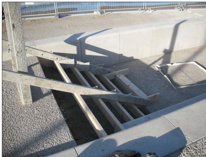
Formwork to stepped access between lower and upper promenade erected ready for concrete to be cast.
