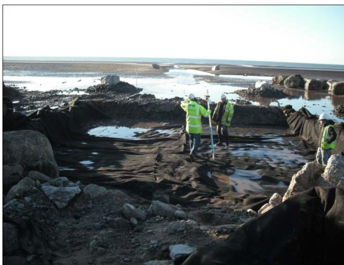
Terminal groyne base excavated and trimmed ready to receive 'rip rap' rock fill.
