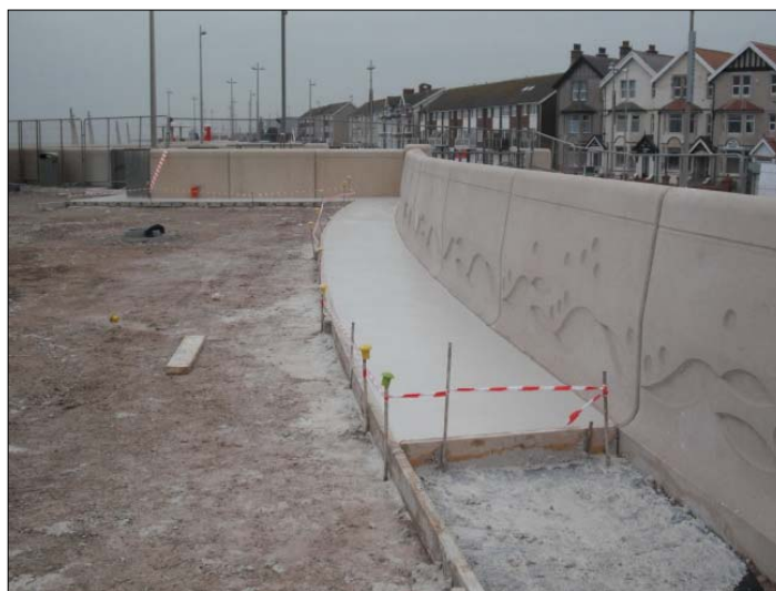
1 metre wide white concrete strip forming part of the promenade pavement adjacent to sea wall.
