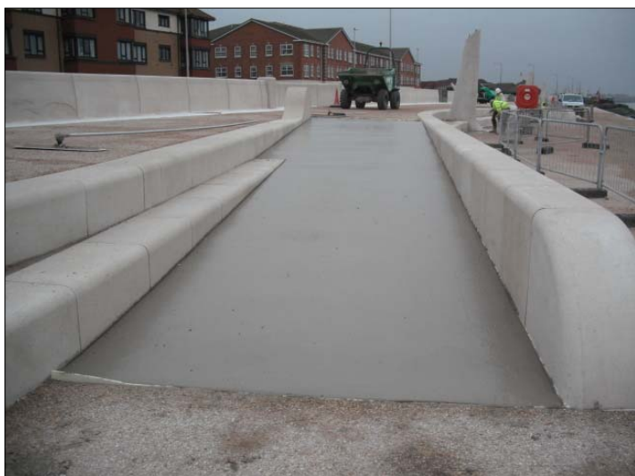
Concrete just placed to one of the ramps between the upper and lower promenade..
