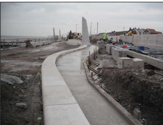
Foundation to upper level of split level promenade intermediate units at wave 2.
