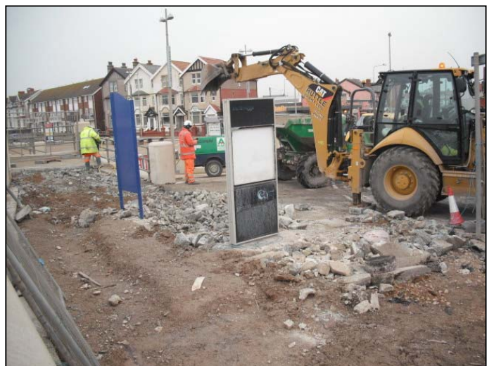
Breaking out works to allow this phase of works to tie in to the completed phase on highway side of wall.
