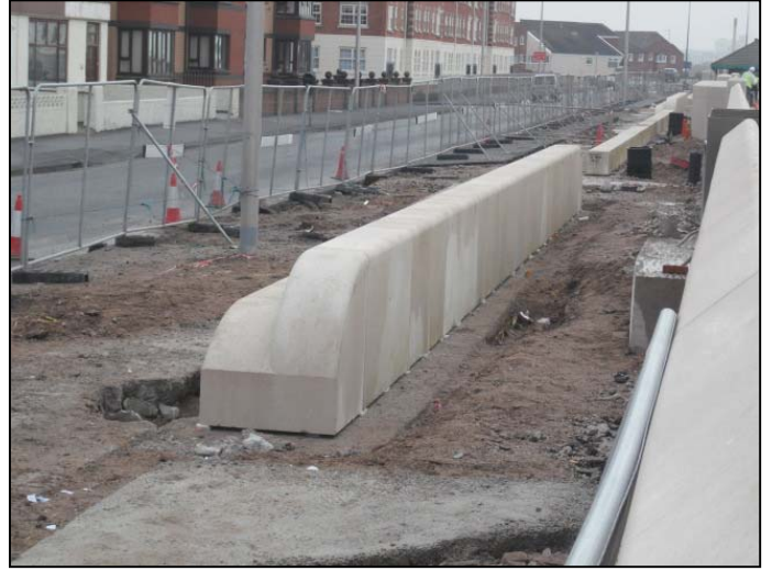
Highway side of completed precast double height intermediate unit to second pedestrian access.
