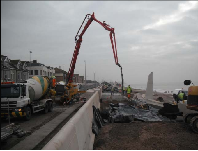
Final section of in situ reinforced base slab to rear walls being poured with the use of a concrete pump.
