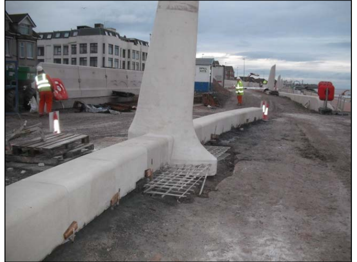
Lower intermediate wall units in place either side of feature lighting column at wave 2.
