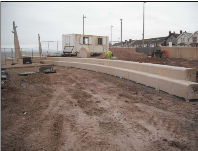
Upper and lower promenade intermediate units in place at wave 1 tying in to completed phase 3 works.
