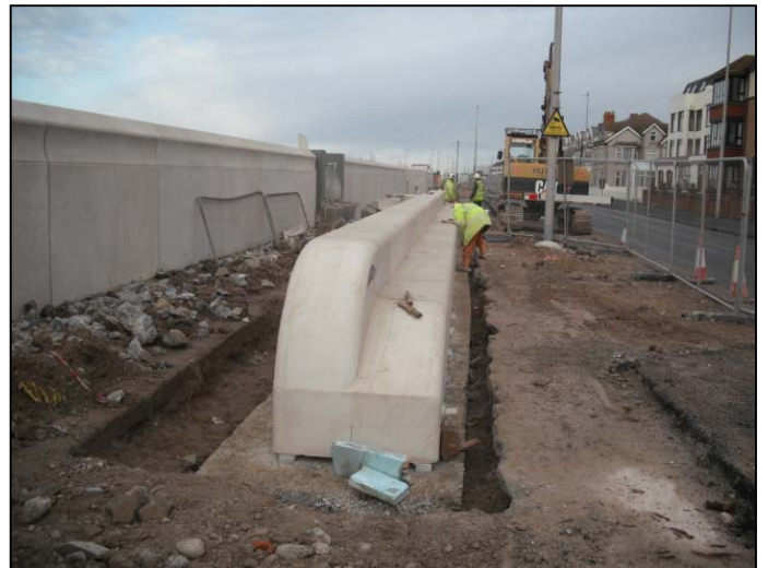
Wall units installed in front of what will be the pedestrian access steps and ramp to the rear wall opening.
