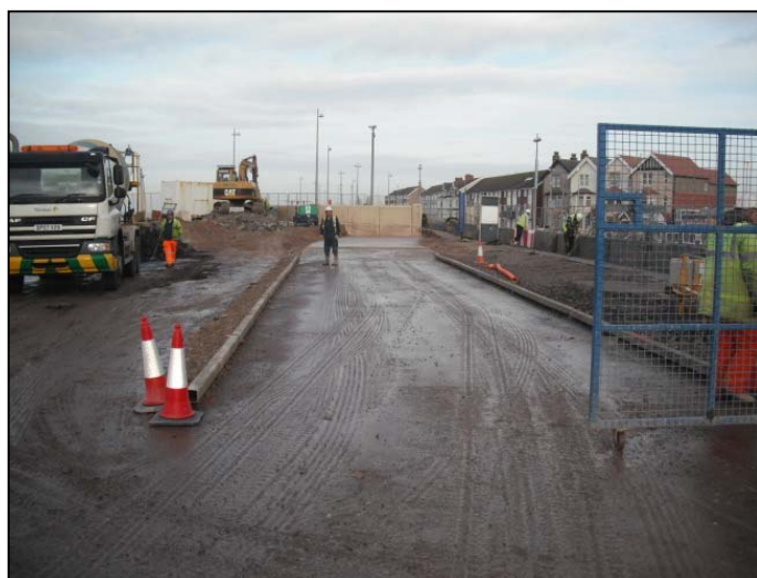
Blinding concrete being placed to form a base from which the rear wall will be constructed
