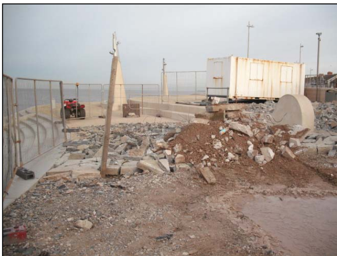
Phase 3 southern most upper and lower promenade sacrificial slabs demolished ready for removal.
