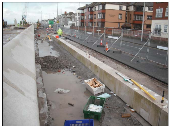
Wall between raised landscaped planting strip and footpath on the highway side of the rear sea wall.
