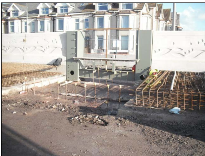
The third and final storm gate frame in place ready for reinforced concrete slab.
