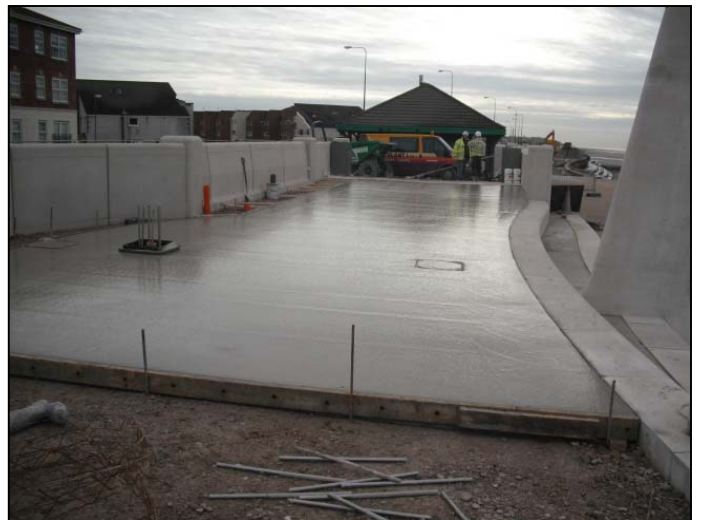
First upper level promenade slab complete reedy for the surface retarder to be sprayed.
