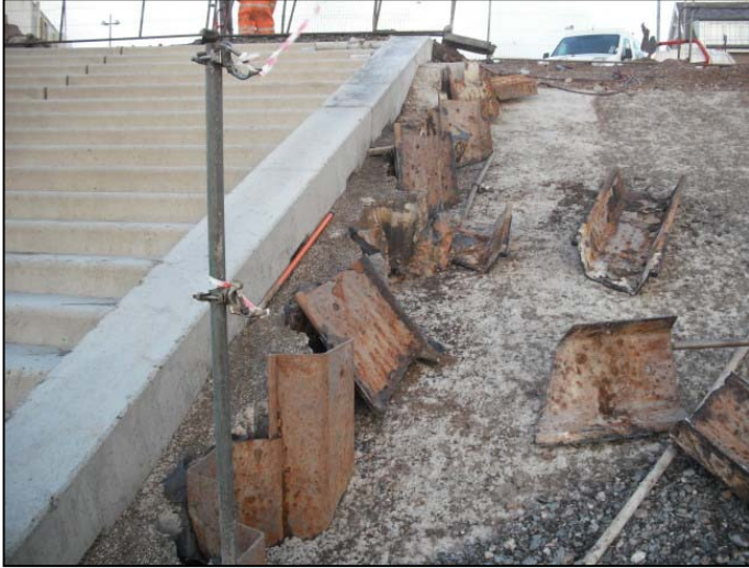
Steel piles and concrete termination of phase 3 being removed to allow last revetment units to be placed.
