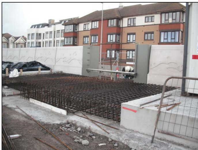
Single leaf storm gate frame and reinforcement in place ready for in-site concrete base.
