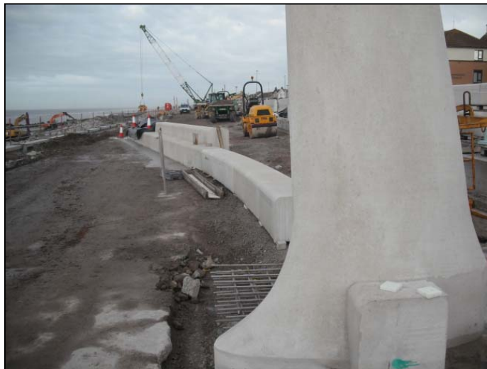
Intermediate walls between upper and lower promenades in place with feature lighting column in the foreground.
