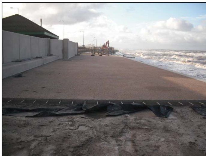
First lower promenade pavement concrete cast with exposed natural golden quartzite aggregate finish.
