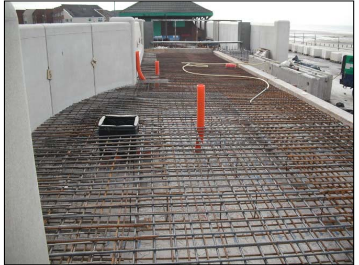
Steel reinforcement to rear walls in place ready for in-situ concrete pour.
