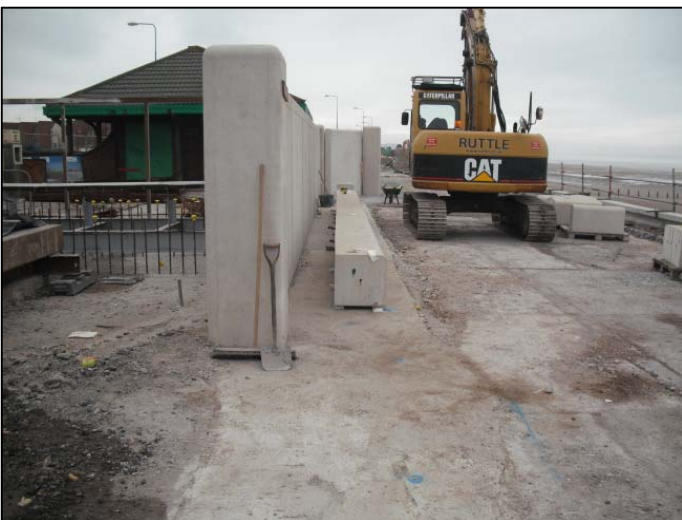
Intermediate pre-cast promenade units being installed to rear of sea wall units around the pumping station.
