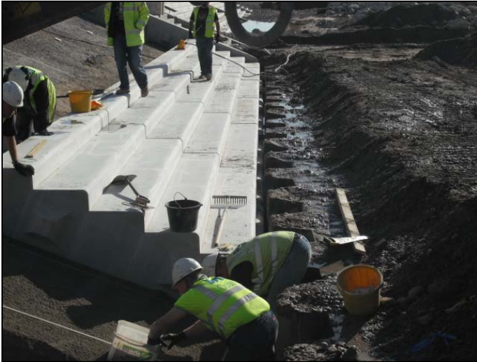
Lower rows of pre-cast revetment units being installed at bottom of panel 3.
