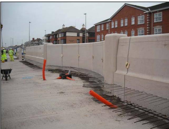
Rear wall units in place ready for reinforcement and in situ base.
