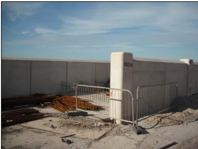
Set back wall and rear wall adjacent to pumping station. This will be the vehicular access ramp and will be the location of the double leaf storm gate.
