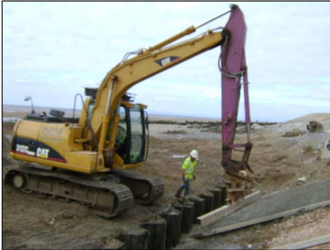
Revetment blinding being levelled off with screed rail adapted for an excavator.
