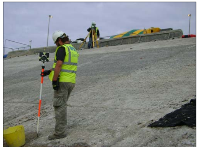
The location of each revetment unit is accurately set by the Site Engineers
