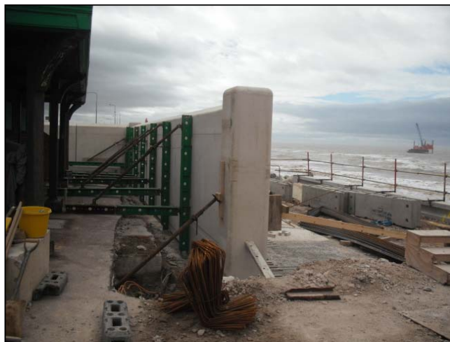
Wall and column units in place and temporarily propped ready for base construction.
