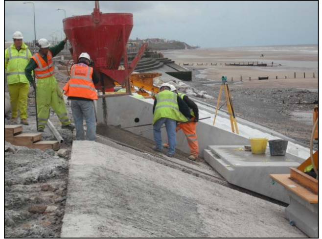
Concrete screed being placed prior to top flight of steps being placed.
