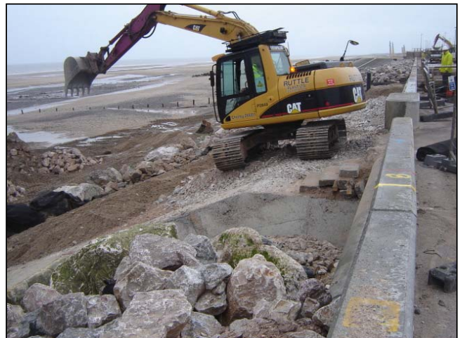
Final central bay of fill material being placed And covered in beach material.
