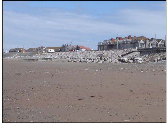
View of the northern half of the filled and loaded revetment area
