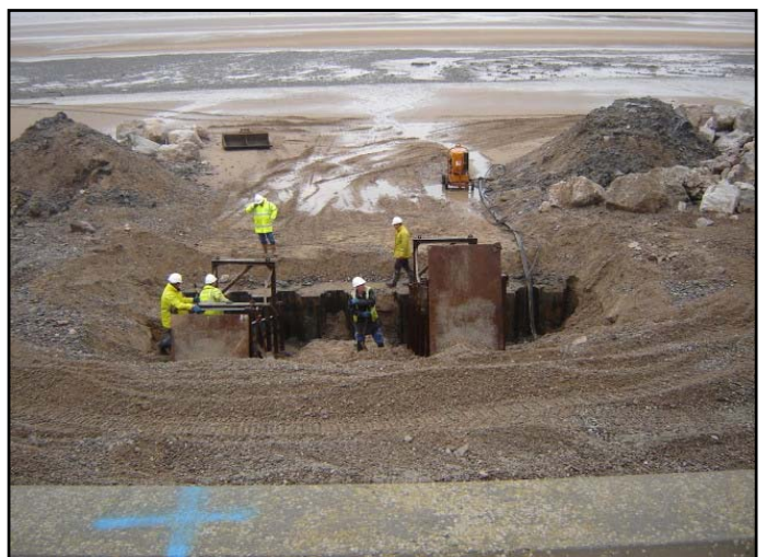
Two lower sections of diaphragm wall being prepared for a concrete pour.
