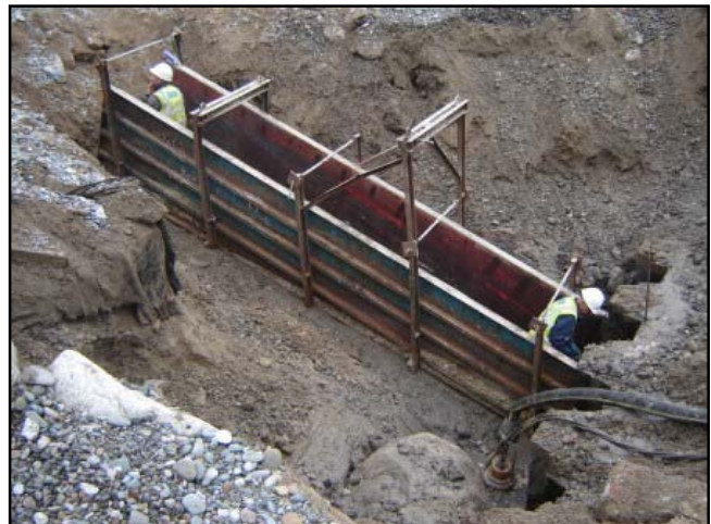
Diaphragm wall formwork being placed ready for a concrete pour adjacent to the toe piles.
