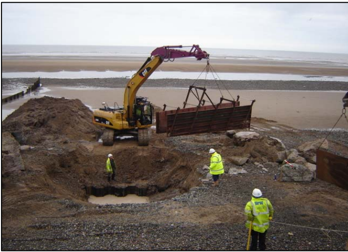
Formwork for lower section of diaphragm wall being placed. Steel sheet toe piles are visible in excavation.
