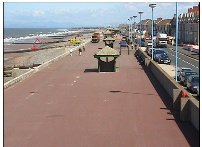
Phase 4 of the works is soon to start south of the existing works
