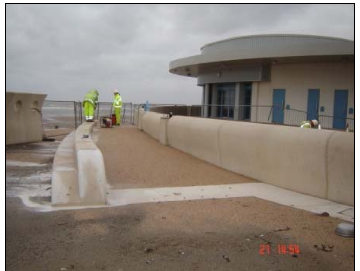
Coring of the café perimeter wall to allow installation of the pedestrian handrailing
