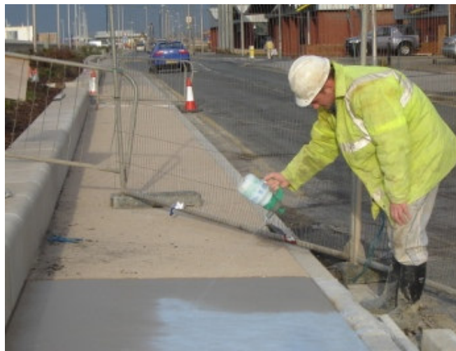
Applying chemical retarder to the new roadside pavement around the plaza area
