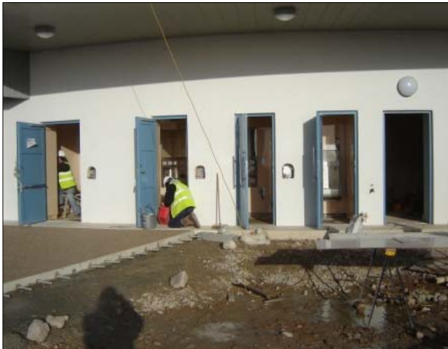
Installation of the toilet facilities. Note the new paving in front of the left toilet doors
