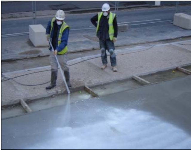
Spraying the concrete retarding agent to the surface of the freshly placed concrete
