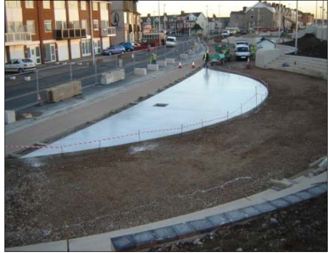
Concreting works to the Children's play area – note the completed footpath next to it
