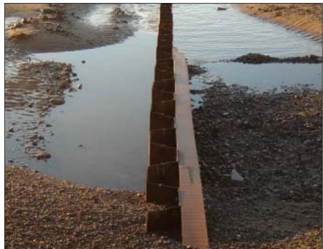
The hardwood timber walings are bolted to the sheet steel pile base
